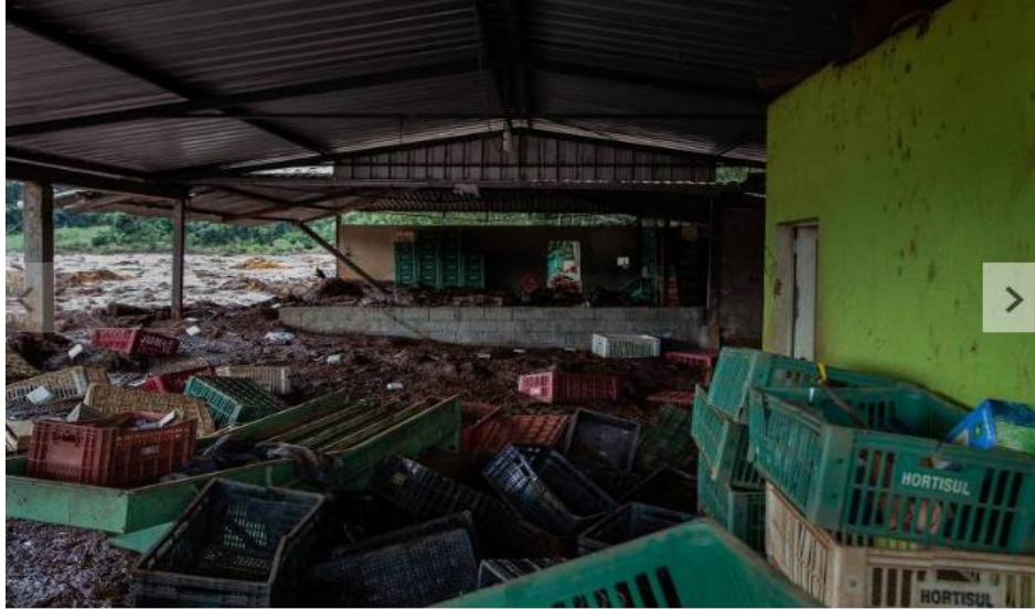
Figure 1: Mud destroyed houses and plantations in the Horta region, which is between Tejuco and Parque da Cachoeira, in Brumadiho (MG). Photo: Eduardo Anizelli Source: Folha de S.Paulo (2019)
